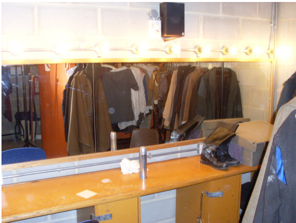
Dressing room lighting to be replaced
